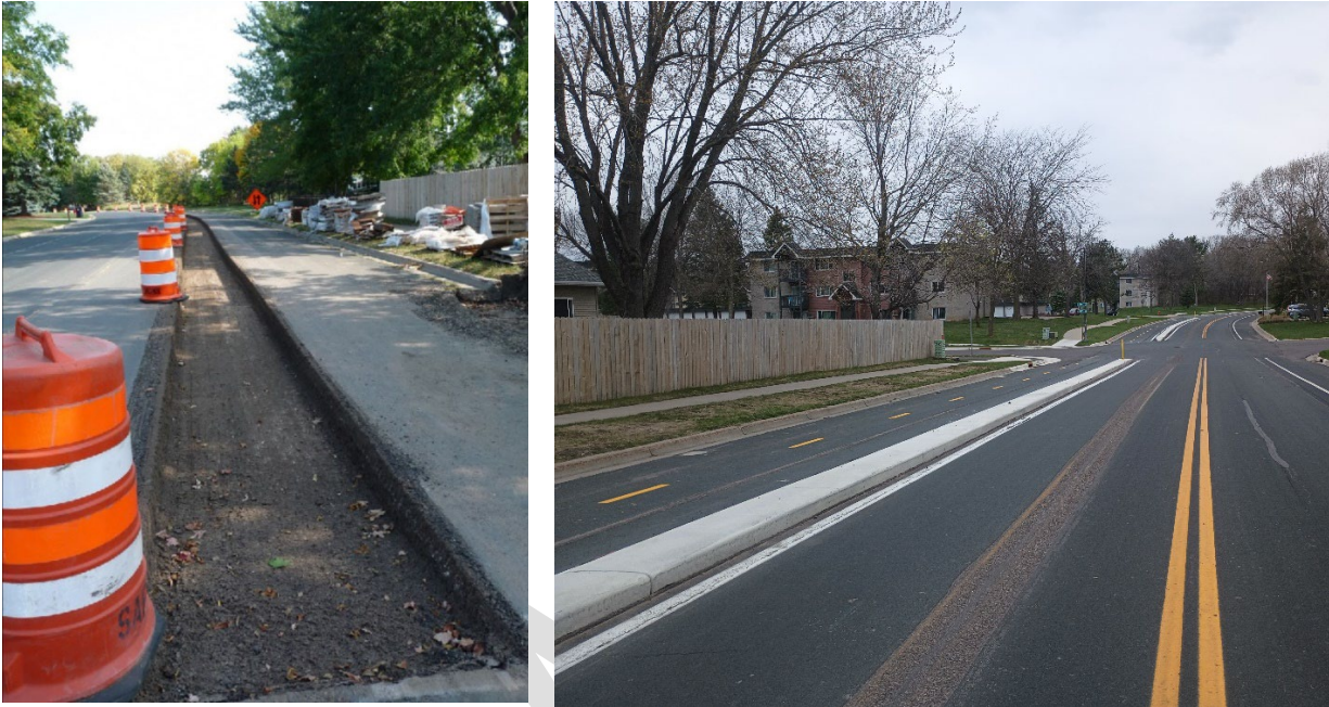
Figure 3.3: Roosevelt Drive in Northfield, MN was recently retrofitted to include a 2-way street-level trail. The facility was created first by saw cutting and removing asphalt (left) and then adding a new curb and restriping the street (right). Left Image Credit: northfieldmnwatchdog.com
