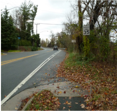
An example of a transition from a sidewalk to a shoulder featuring a detectable warning surface.
