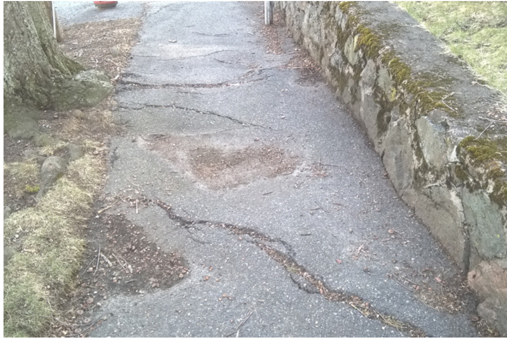
An example of a sidewalk that has become degraded over time due to deferred maintenance.
