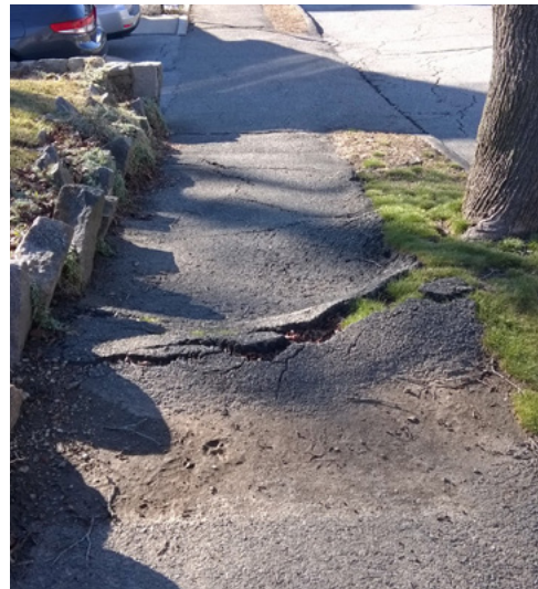
An asphalt sidewalk with root damage.
